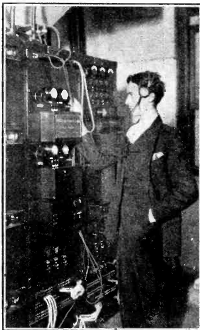
HOTEL WIRELESS. 2,200 rooms in the Pennsylvania Hotel, New York, are now equipped with broadcast receiving "points." The switchboard seen in the photograph distributes programmes throughout the rooms and also controls the transmission of programmes from the hotel.
